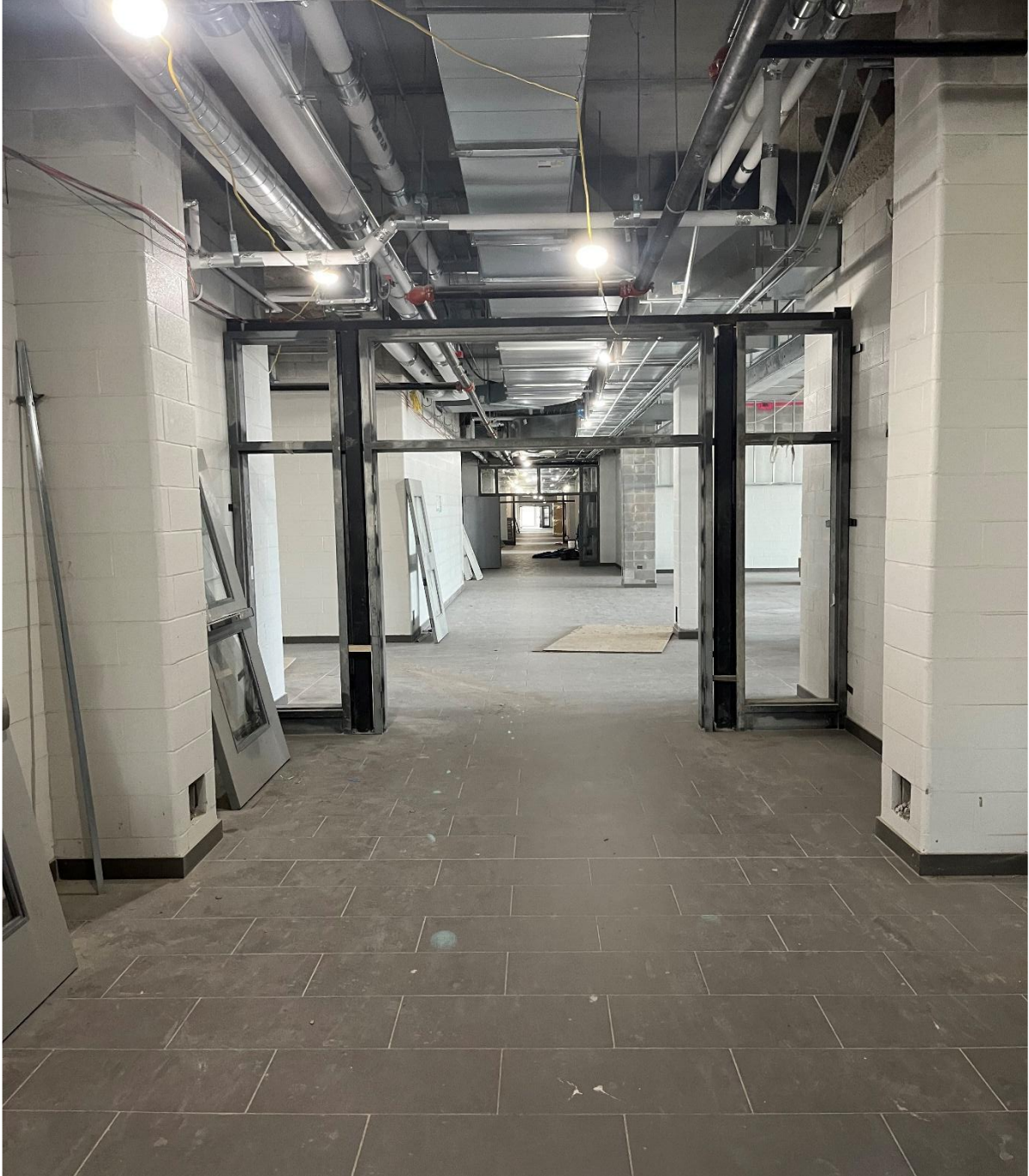
Finishing work, such as MEP, doors, painting and flooring, is currently underway in the corridor."
