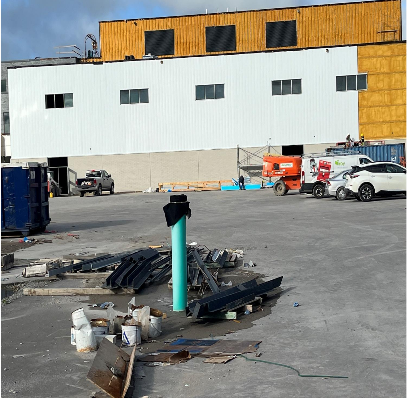
Ongoing installation of metal siding panels with a view on the east elevation
